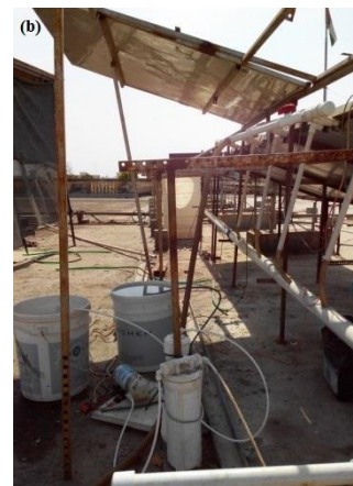
Fig. 1. (a) Photovoltaic panels kept at 20° inclination from horizontal; (b) RO plant associated with PV panel.
