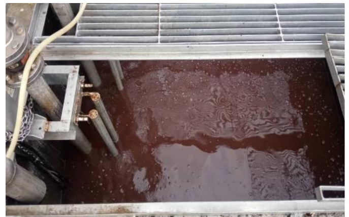
Fig. 1. Sump inlet used to collect the wastewater from the slaughtering and cleaning process.
